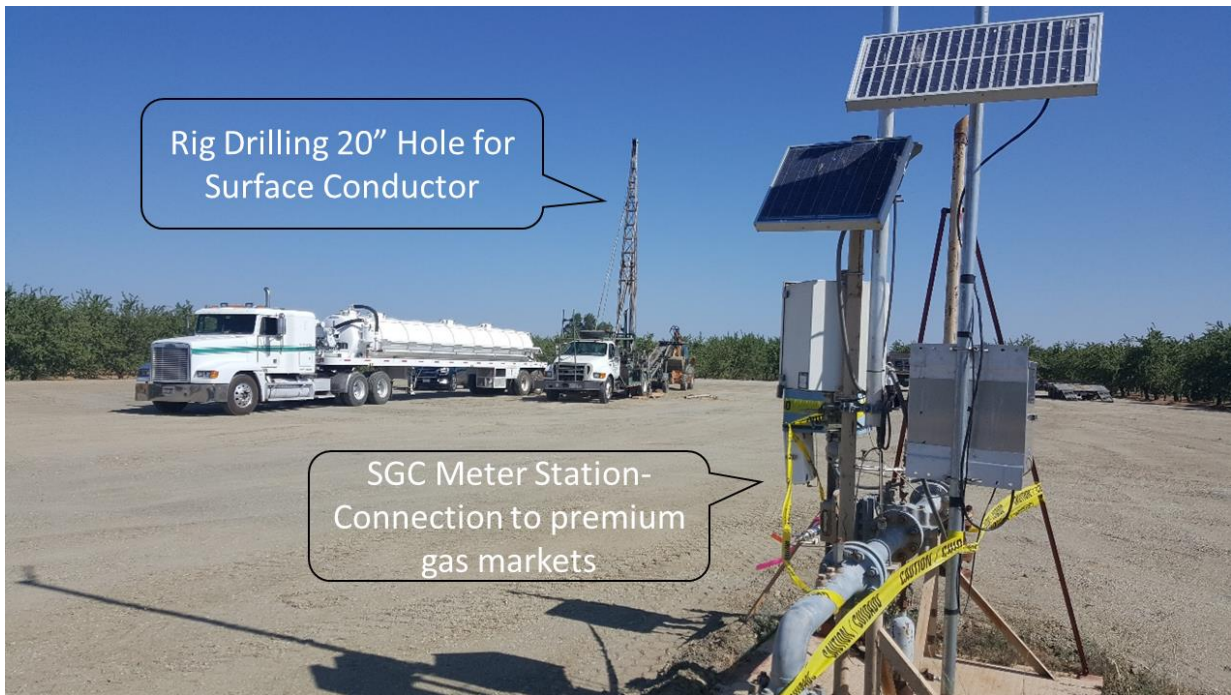
Figure 2: SGC Gas Meter and Surface Conductor Rig
