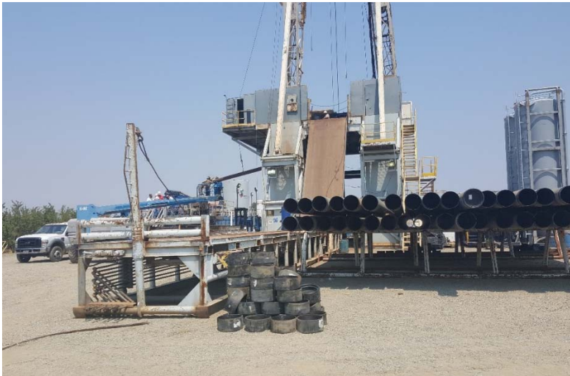
Figure 1: Casing ready for running at Dempsey 1-15 Natural Gas Well, Sacramento Basin, California
